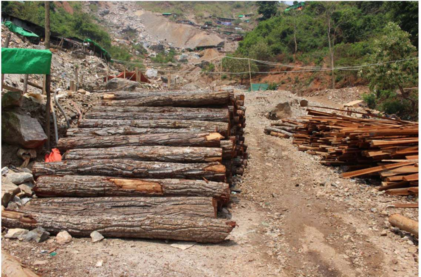
Figure 21 the company and small-scale mining operators systematically collect logs to be used as supports, reinforcing the roof and maintaining the structural stability of the tunnels in the dimly lit, confined environment
