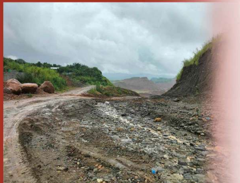
Figure 9 A picture showing how a village road was damaged and destroyed due to jade mining operations.
