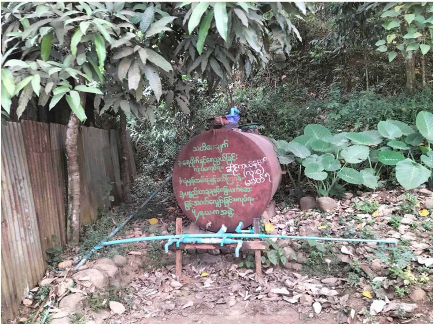
Figure 3 Water tank for distribution to households.
